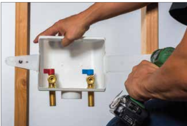
Installation Difficulty. Flimsy box and brackets require extra work and leveling to install correctly.
